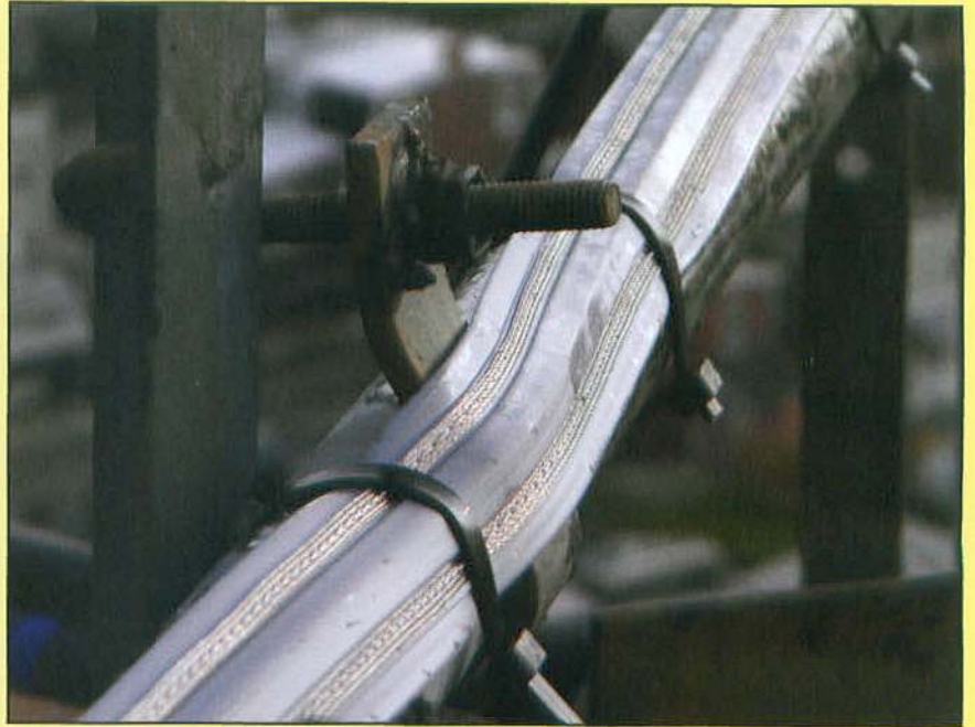
This close-up shows the electrified track as attached with plastic grips. Glue normally is used, but a previous application of a sticky substance intended to deter the birds prevented the use of glue to attach the tracks here.
